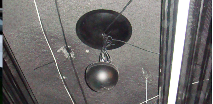
Installed transducer with acoustic disc
